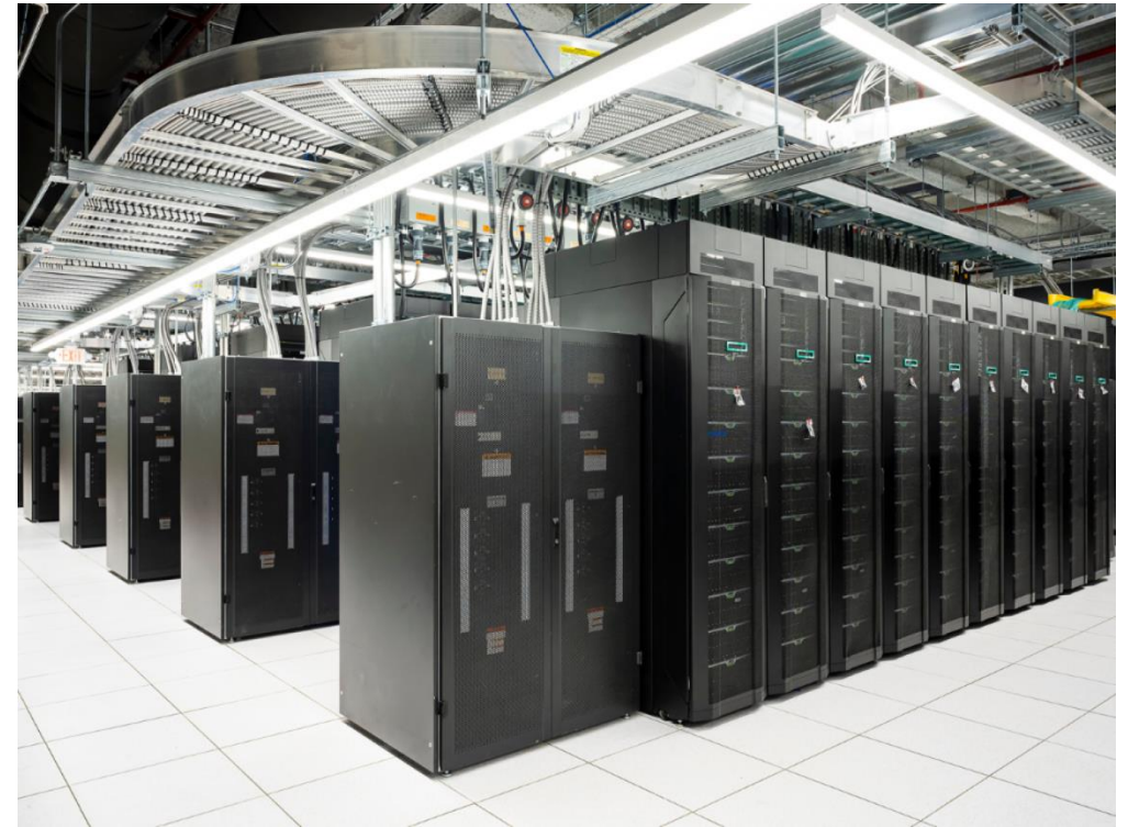
SMRs & Data Center-DOE Report-2025
